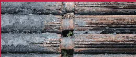
Used longitudinal coils showing significant coking.
